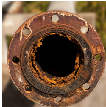
ID of corroded pipe sample
